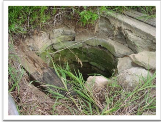
Picture of a hazardous abandoned well
